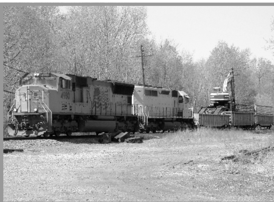
Spring is bringing major work projects to CSX's Henderson Sub. Ron Stubblefield caught this CSX work train unloading ties at Nortonville on April 8. There are ties and fresh ballast on or near the tracks from Nortonville south to Hopkinsville. The crews should be working on the tie replacement any day now. digital image by Ron Stubblefield
